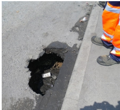
Collapse in Carriageway
