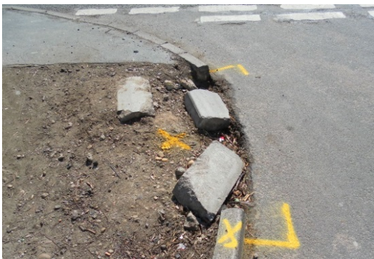
Loose or missing kerbs
