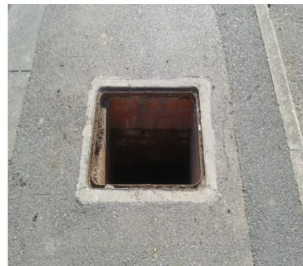
Missing Manhole Cover
