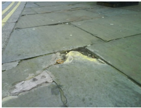
Level difference to broken/damaged flags
